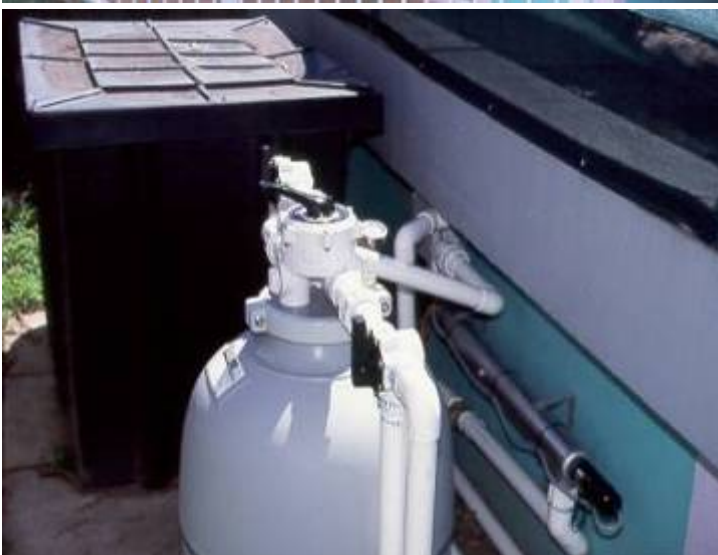
Three types of filtration- Mechanical (Grey pond filter), Biological (black tub with dense matting) and UV Clarification/Sterilisation (Stainless steel tube)
